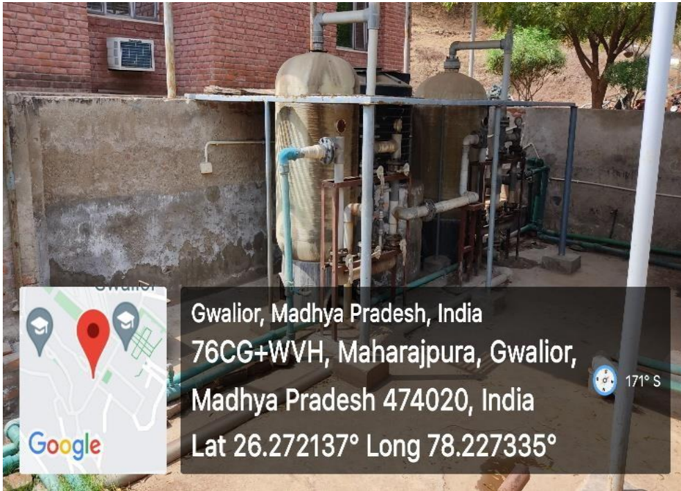
Water SoftnerNear Chillar Plant
