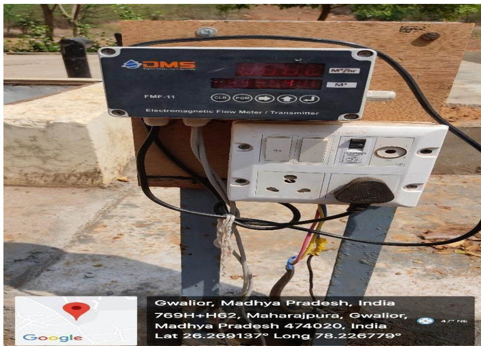
Water Meter Behind C Block
